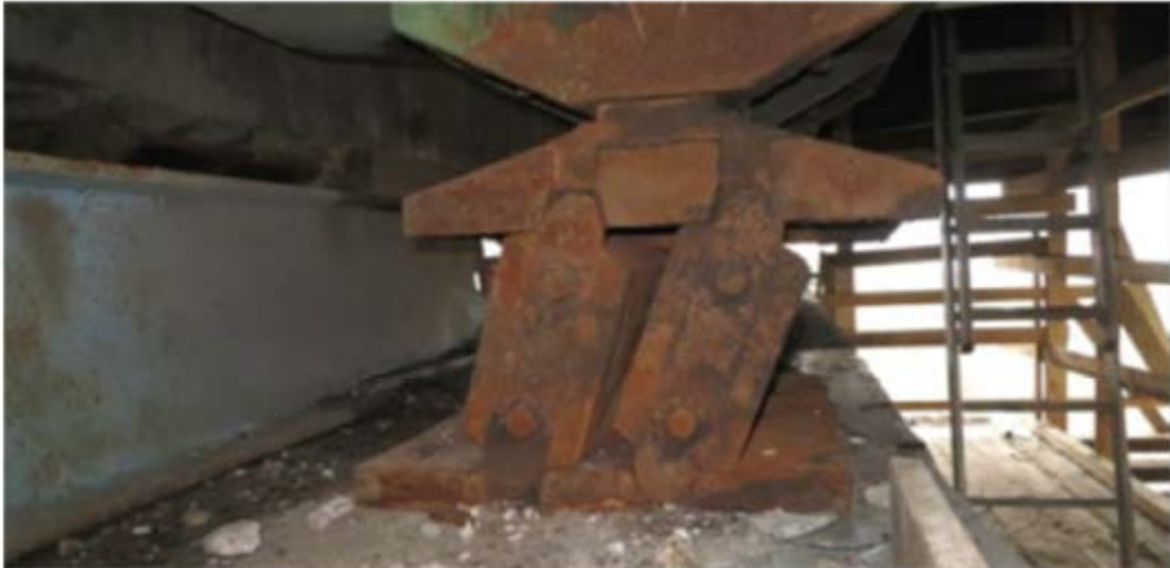
A displaced bearing on the edge support of Łazienkowski Bridge
