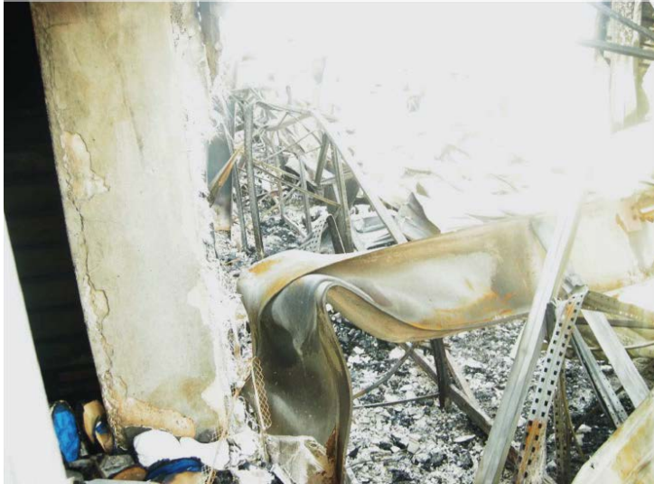
View of a portal frame column subjected to fire [51]
